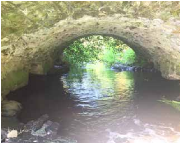
Pict 2.7 Scour damage on Ballygrogan Bridge
