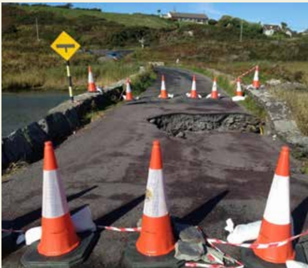
Pict 2.3 Damaged road before temporary bridge
