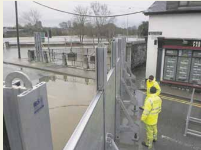
Pict 2.6 Demountable defense during flood event
