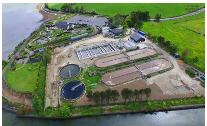
Clonakilty Waste Water Treatment Plant
