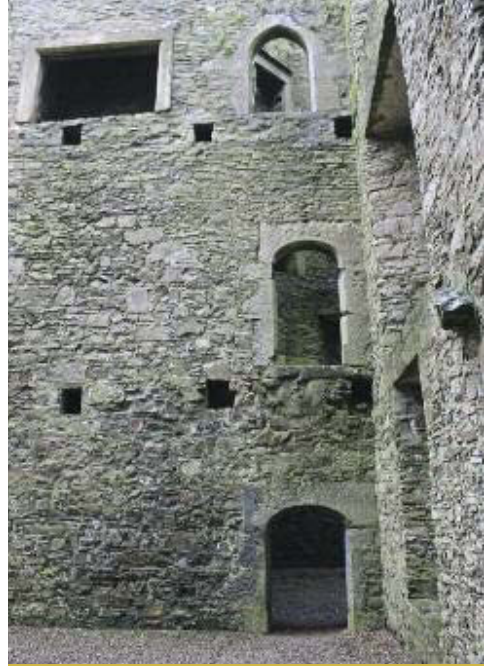
Interior doorways at Kanturk Castle. The uppermost has the pointed, Gothic arch harking back to the medieval period. The flatter arches on the others are typical of the late sixteenth and early seventeenth centuries.
