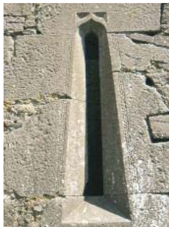
Ogee headed ground floor window at Ballinamona Castle using chamfered edged limestone blocks dressed with subtle pick dressing.
