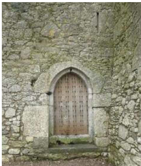
The entrance door to Barryscourt Castle. Note the 'yett' holes at the apex and left side of the doorway. An iron grille hanging outside the door was secured by passing chains through the holes and securing them inside.
