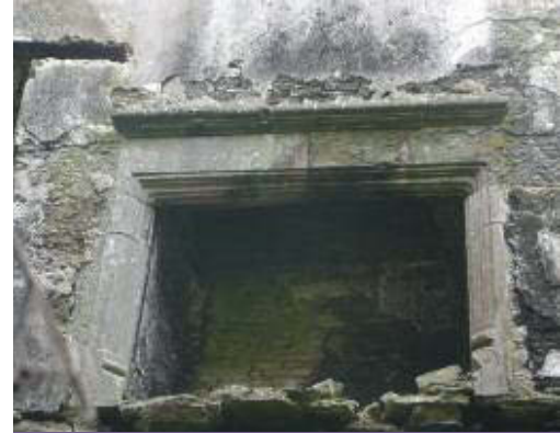
ABOVE: Fireplace at Ightermurragh Castle. The flat lintel and the moulding along the edges are typical of the seventeenth century.
