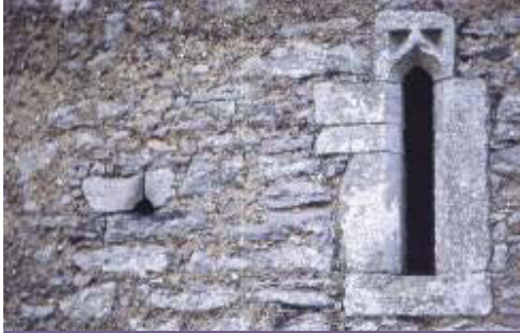
Ogee head window at Carrigabrick Castle, Fermoy made from dressed limestone blocks with chamfered edges and decorated with hollowed out spandrels, it is flanked by a gun loop to the left.
