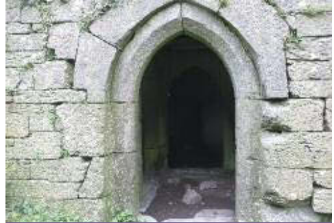
The pointed arched door at Kilcrea Castle using dressed limestone with chamfered edge leading into the entrance lobby. Image by Eoghan Nelligan.
