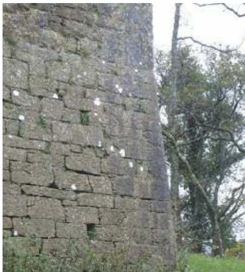
Base Batter - note how the wall thickens as it approaches the base.
