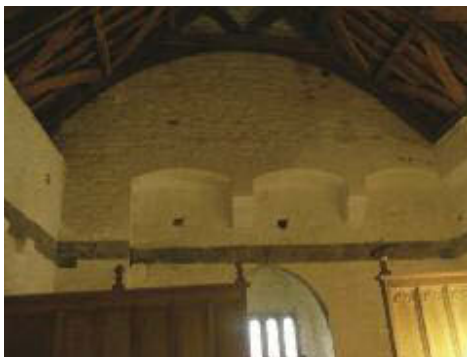
Arcading in the Great Chamber of Barryscourt Castle. The roof is a modern reconstruction.
