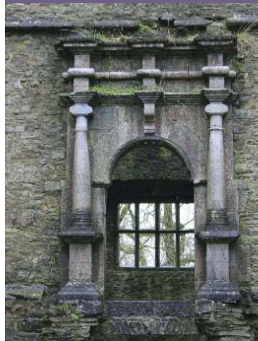
BELOW: Renaissance-inspired entrance doorway to Kanturk Castle. It is constructed of cut and dressed limestone and consists of a round headed arch framed with classical pilasters that support a banded frieze and cornice.
