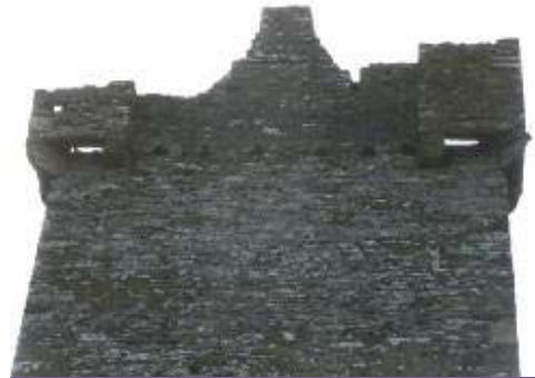
ABOVE: Corner bartizans on Castledonovan castle. The row of holes in the wall between the bartizans is to allow rainwater from the roof to run off.
