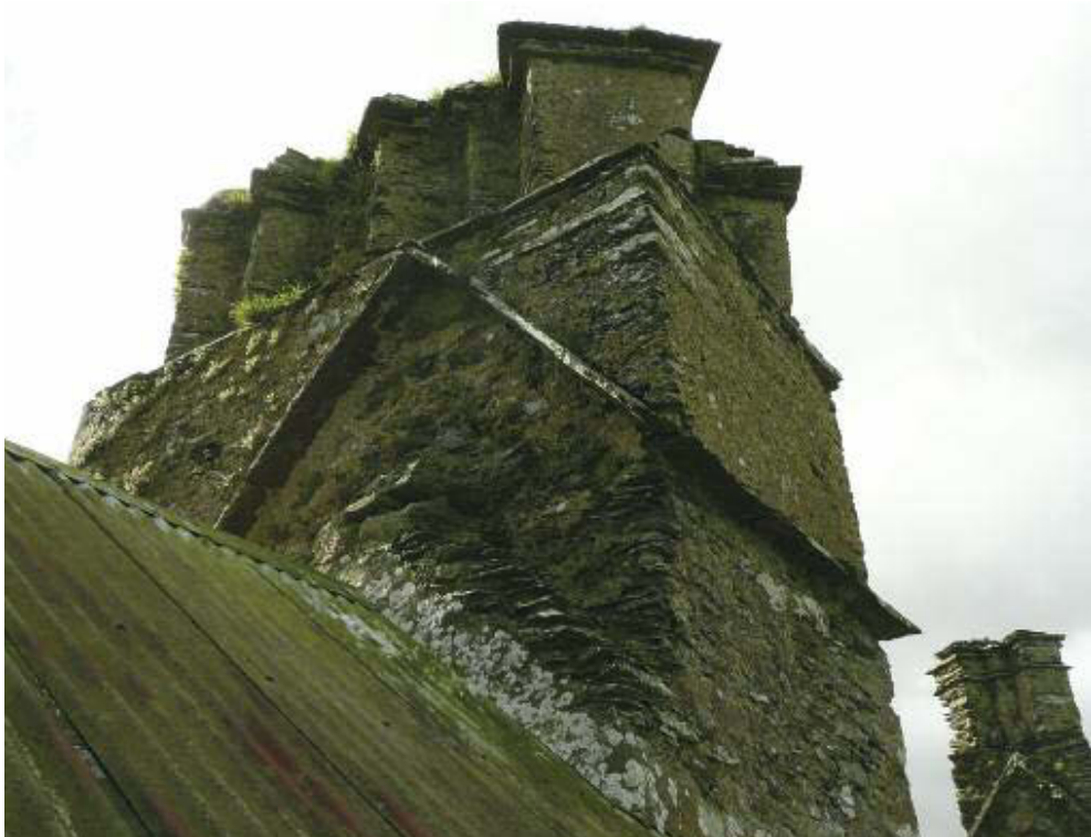
Togher Castle chimneys. Note projecting stone flashing for original roof and diagonal 'Jacobean' chimney pots. The corrugated iron roof was installed in the early 20th century.
