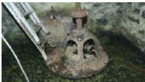
The American water turbine at Castleview Mills, installed originally in 1918 and still working.
