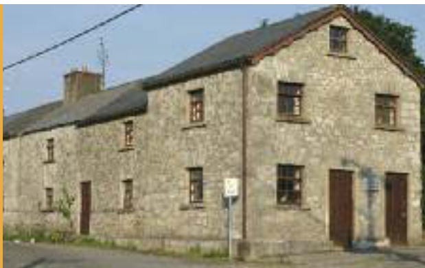
Early nineteenth century workers' housing at Ballincollig Gunpowder Mills, known as the Long Range.
