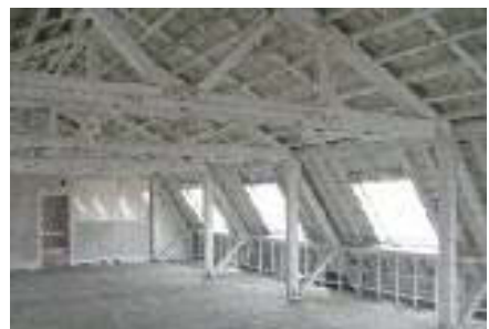
Baltic pine used for roof trusses, stanchions, and floors in former British Naval storehouse on Haulbowline Island, Cork Harbour, c. 1818.
