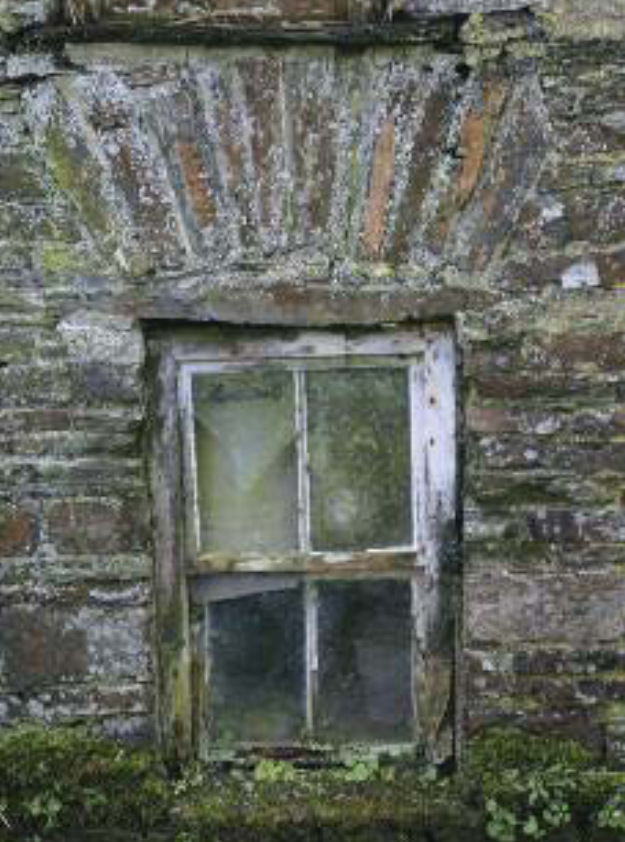
Late eighteenth-century, using the combination of stone lintel under an arch at Castleview Mills.
