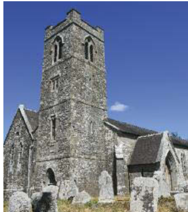
Kilshannig Church, near Mourneabbey. Built of random rubble limestone with cut-stone detail.
