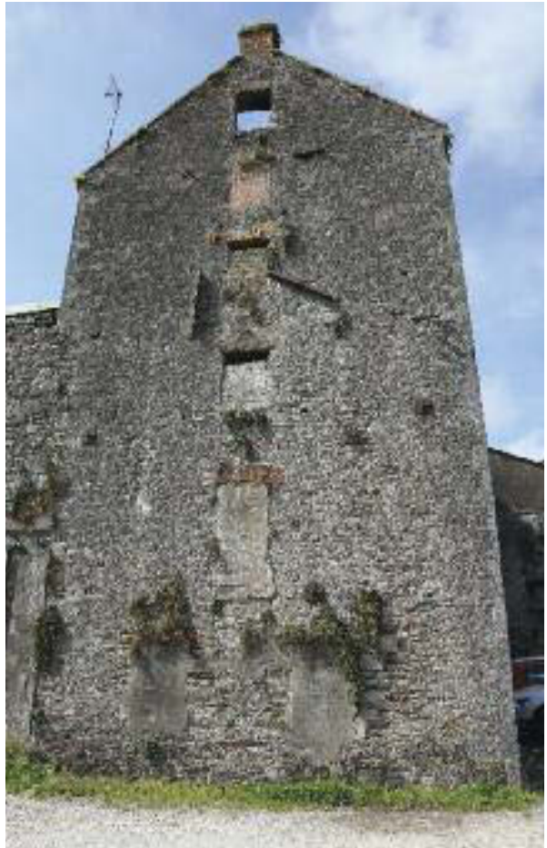
Killeagh Mills, west gable of main buildings. Note the use of tie plates to prevent external wall of building from buckling outwards under the weight of grain formerly stored on upper floors.
