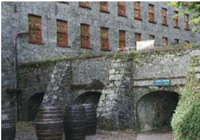
Stone aqueduct carrying the mill race to the high breastshot suspension waterwheel of 1852, at Midleton Distillery.
