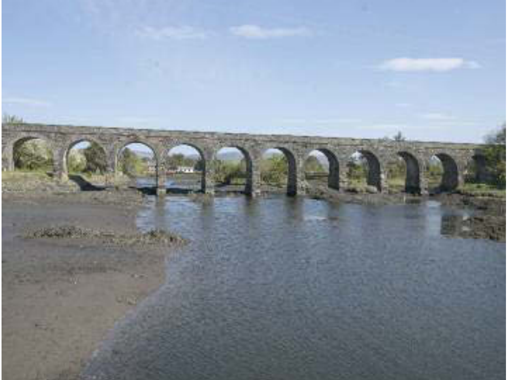
The Ballydehob viaduct, which carried the Schull and Skibbreen line over an inlet of Roaringwater Bay, completed in 1884-6.
