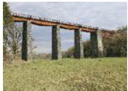
The Carrigabrick viaduct (1872) which carried the Fermoy-Lismore line over the River Blackwater near Fermoy.
