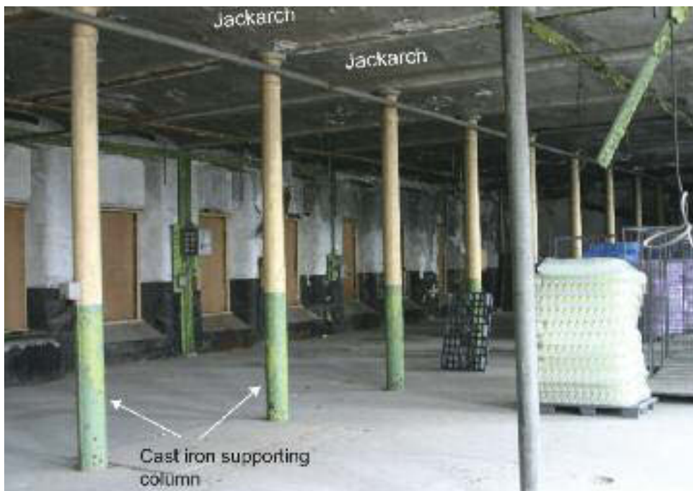
Internal cast iron framing and jackarch fireproofing in former Lansdowne flax-spinning, Limerick, built in 1853.
