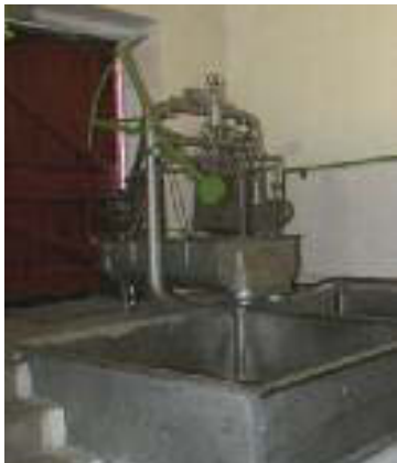
Large steel weighing pan at Emly Creamery, county Tipperary. The loading door can be seen in the background, which would have had a ramp or stepped platform to facilitate the lifting of the heavy milk churns from carts.
