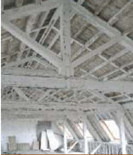
King post truss roof in former British Naval storehouse on Haulbowline Island, Cork Harbour, c. 1818 (Exemplar 25).
