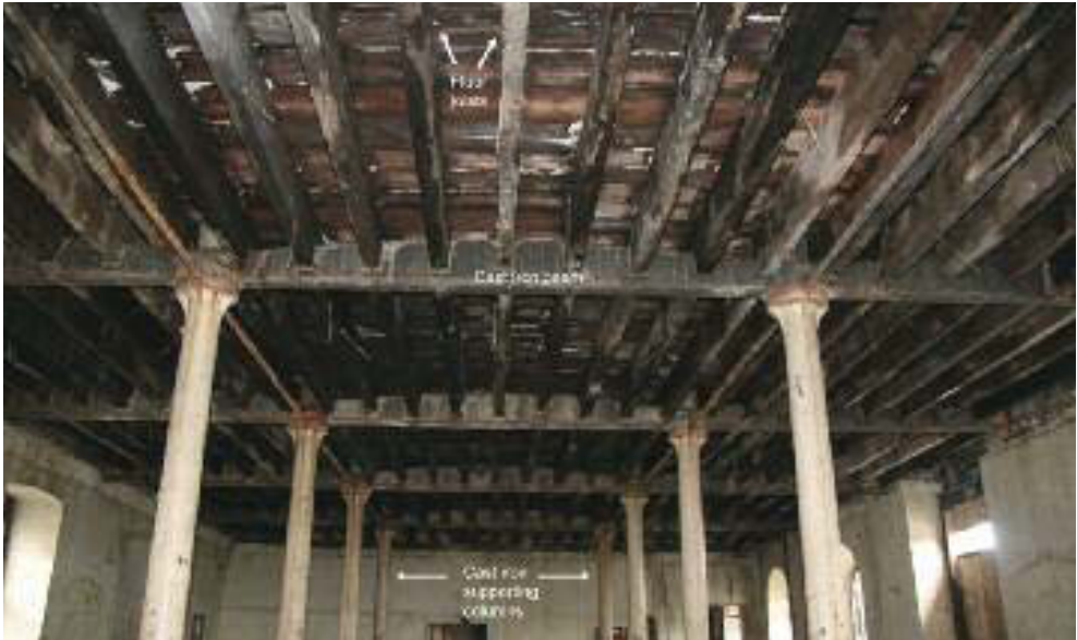
Internal cast iron framing in former British naval storehouse on Haulbowline Island, c.1816-22.
