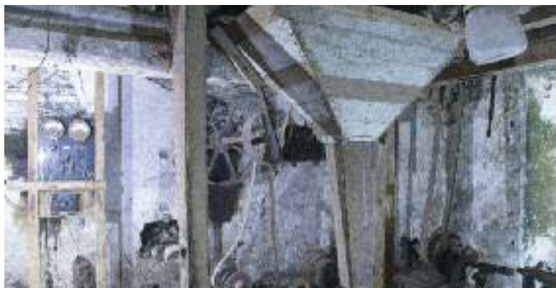
Control panel for electricity generating set, installed in Castlevew Mills in 1918.
