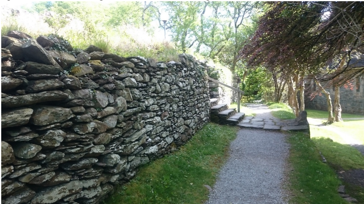
Figure 7.3 Bulge in wall visible on left of image
