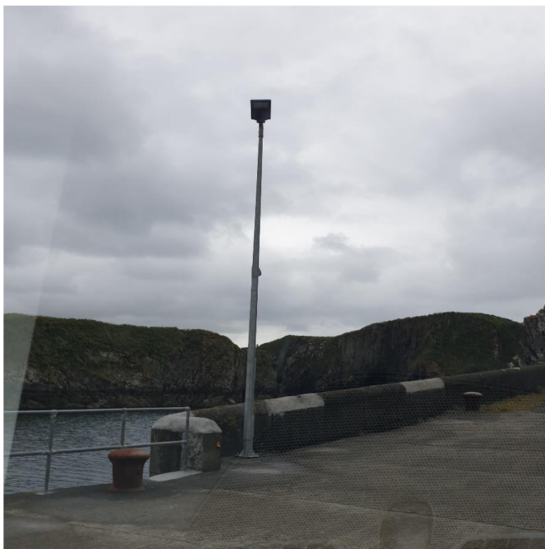
Integrated solar powered light recently installed at Kilcrohane Pier.
