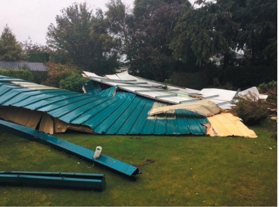
School Gymnasium, Douglas after Storm Ophelia. Source: Mona Lynch
