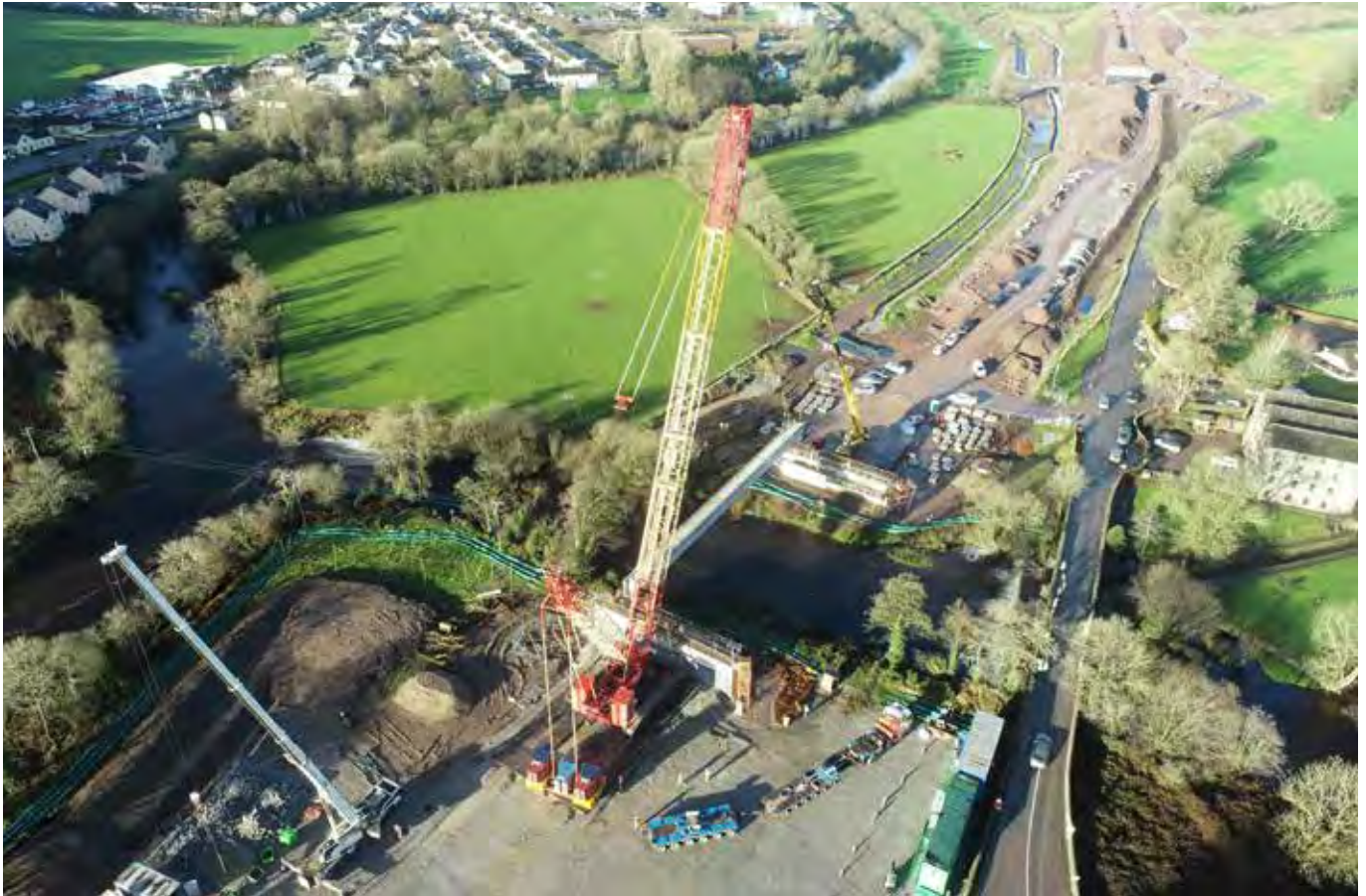
Construction advanced on the N22 Baile Bhuirne to Macroom Road Development in 2020
