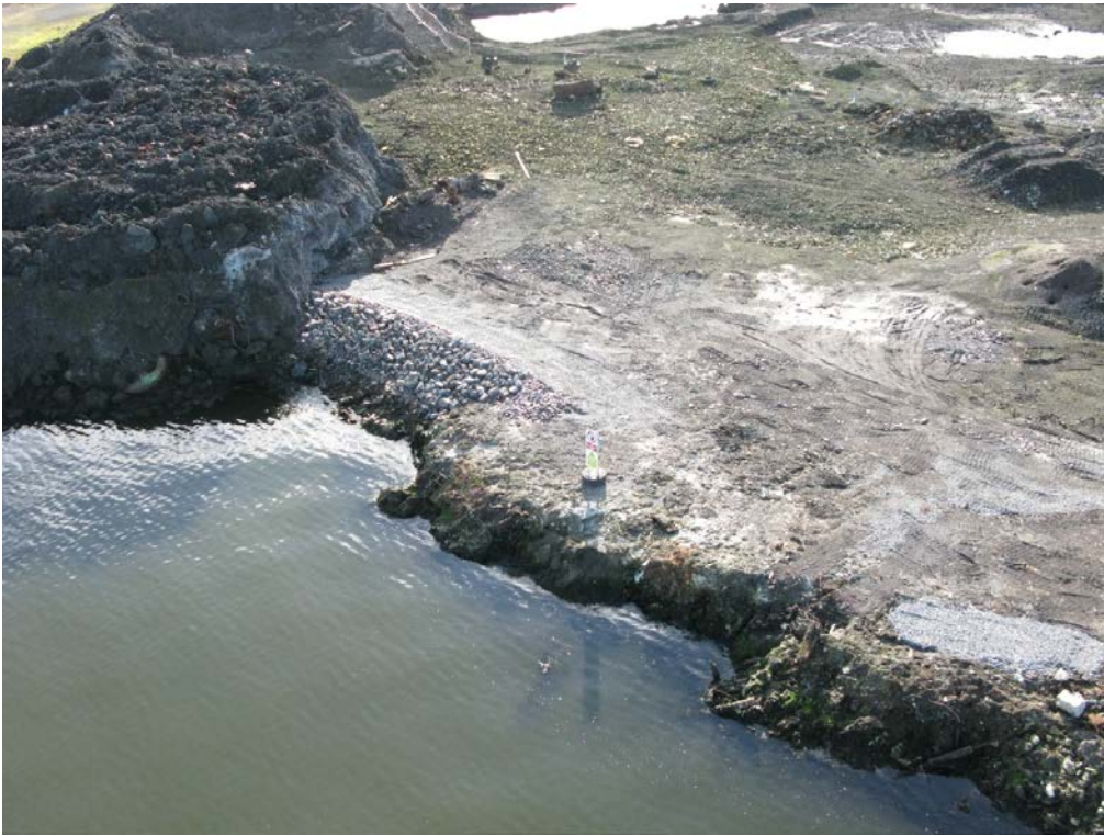
Plate 5 Aerial photograph showing repair of eastern sea breach. (Courtesy of SkyTec Ireland)
