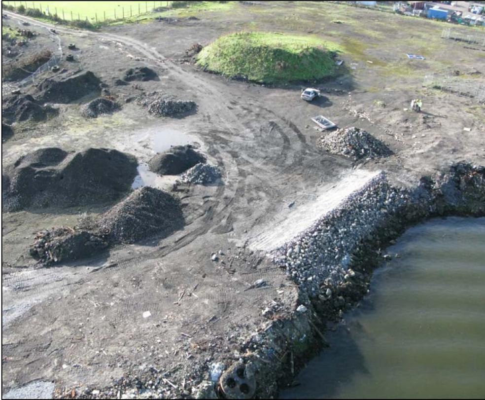
Plate 3 Aerial photograph showing repair of western sea breach. (Courtesy of SkyTec Ireland)
