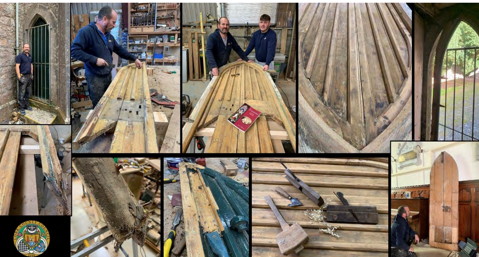
Restoration works of the 190 year old vestry door at St Georges Heritage and Arts Centre. The repaired door will allow for a second entrance to St Georges for when restrictions ease to allow visitors.
