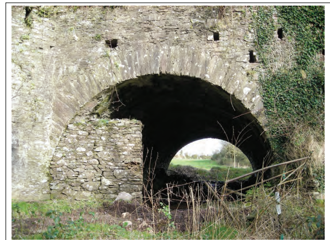
Right: 'Dry' left hand arch proposed as pedestrian link under Old Mallow Road, connecting the 3 northern villages to the Country Park.
