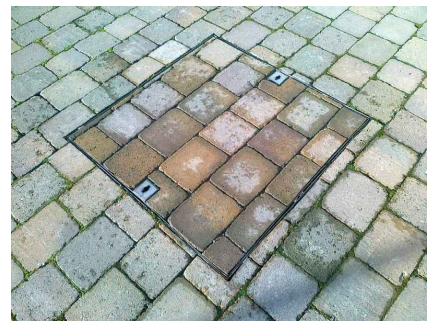
Sample of Recessed Manhole Cover
