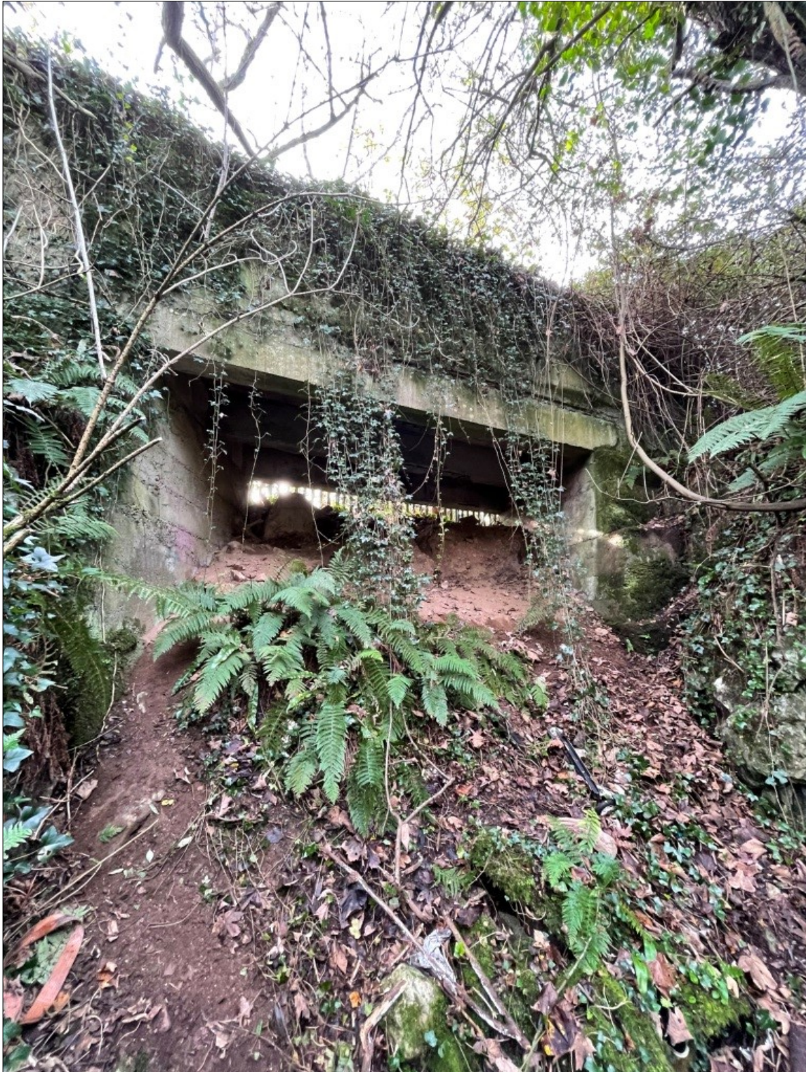
Plate 1: View to overpass from within cutting with the ground below having been infilled.
