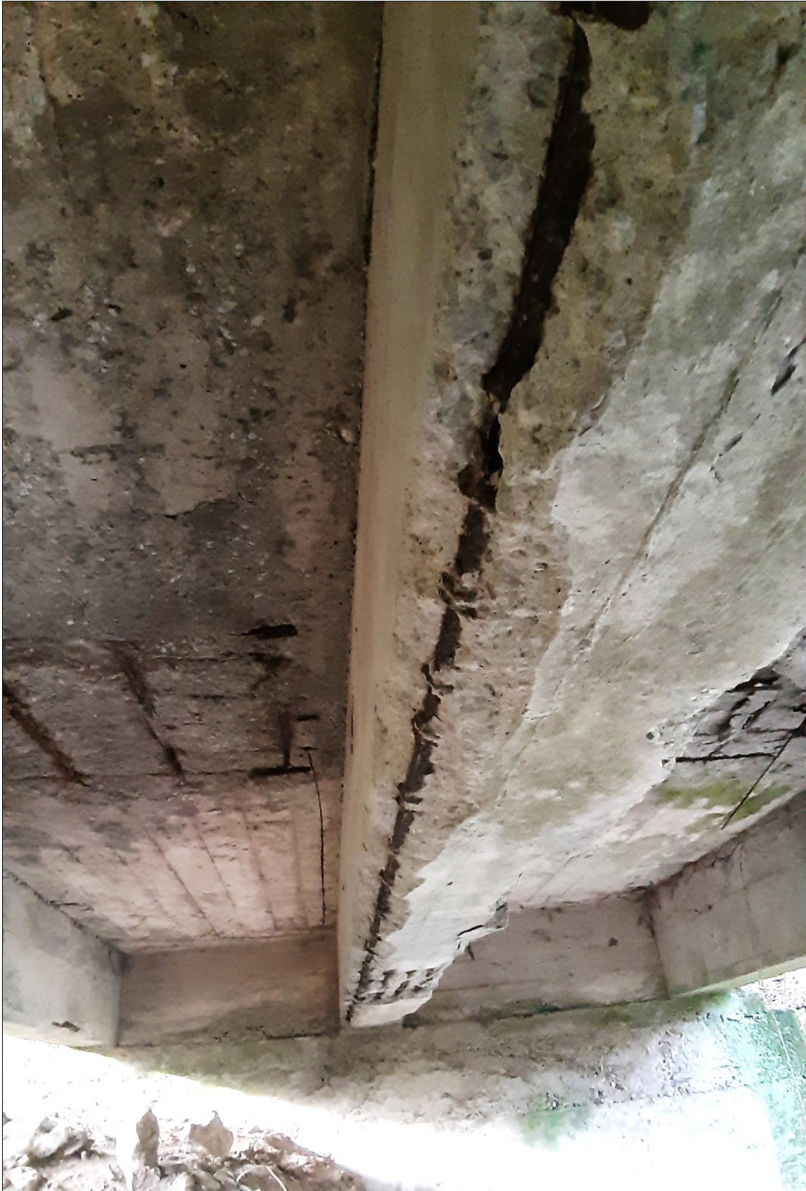
Plate 5: Decayed concrete and exposed reinforcement bars
