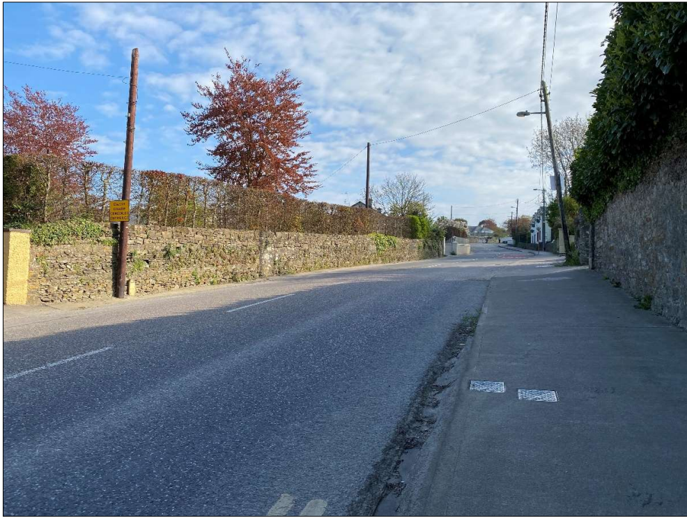
Plate 11: Section of random rubble wall (CHS 11) on the eastern side of Church Hill
