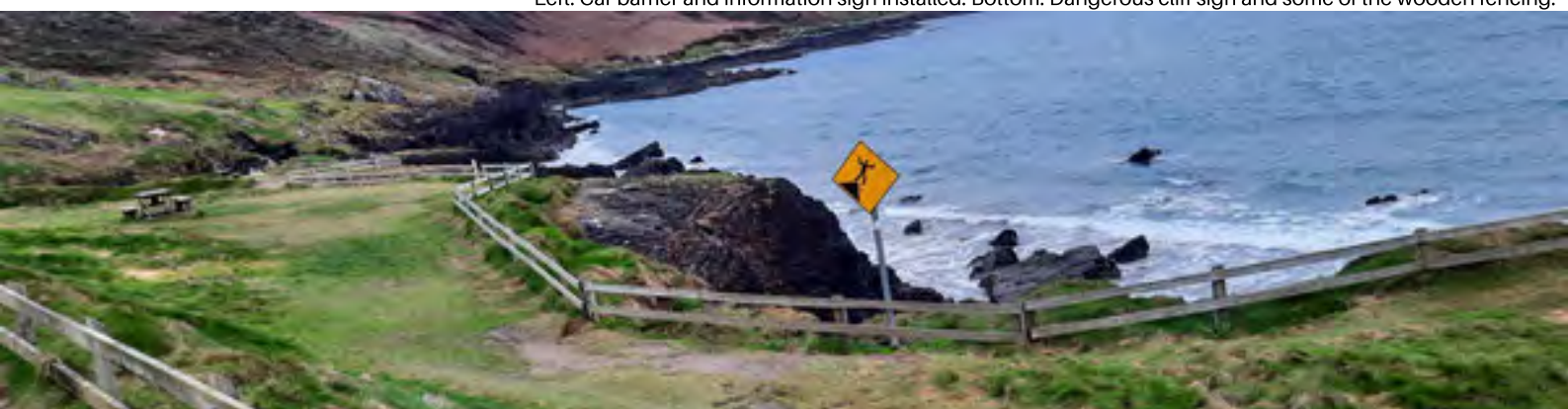
Left: Car barrier and information sign installed. Bottom: Dangerous cliff sign and some of the wooden fencing.
