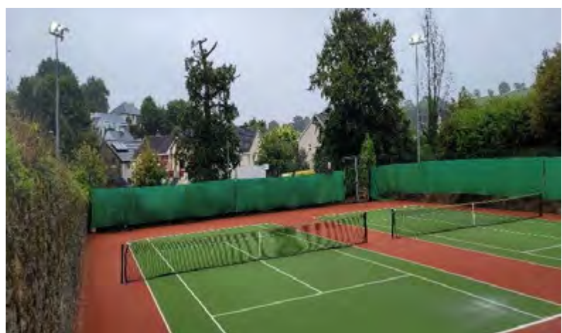
Upgrade of existing floodlights to LED lighting at Crosshaven Tennis Club, completed with the support of 2021 Amenity Grant (right).
