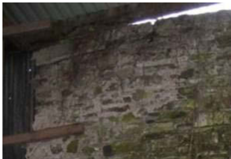
Plate 88: Damaged upper level of wall
