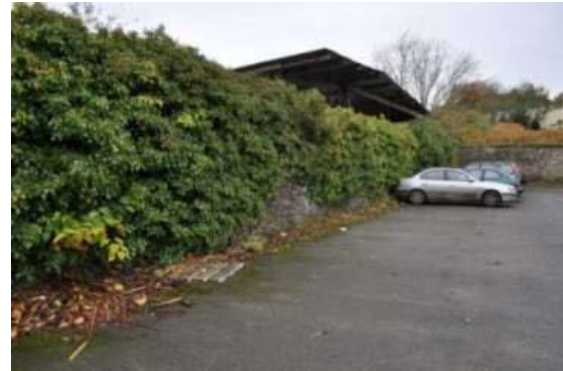
Plate 40: East elevation of town wall forming boundary to P.O. yard, looking north-northwest.
