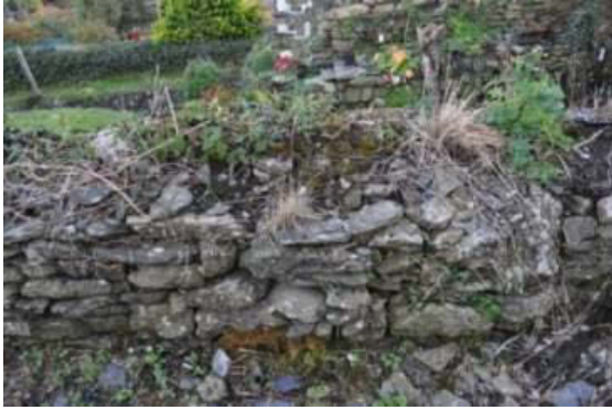
Plate 49: Line of town wall forming plot boundary at rear of O'Brien's property, looking south-east.
