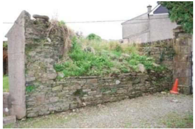
Plate 19: Possible defensive feature at south-west corner of town wall within St Peter's graveyard, looking south.
