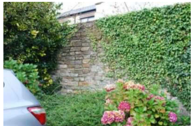
Plate 5: Modern rebuild of east (internal) elevation of Section 2 from Garda Station car park, looking west.
