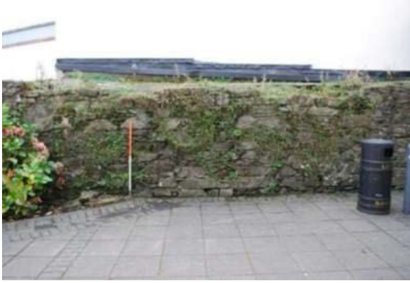
Plate 9: Possible original portion of original wall face (west elevation) at south-west end of Section 2.
