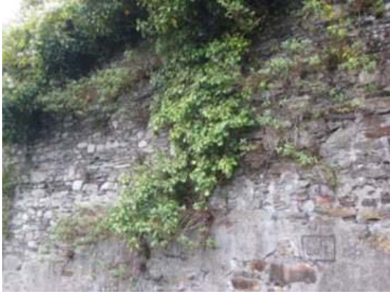
Plate 73: Cementitious render to wall with plant growth along the top
