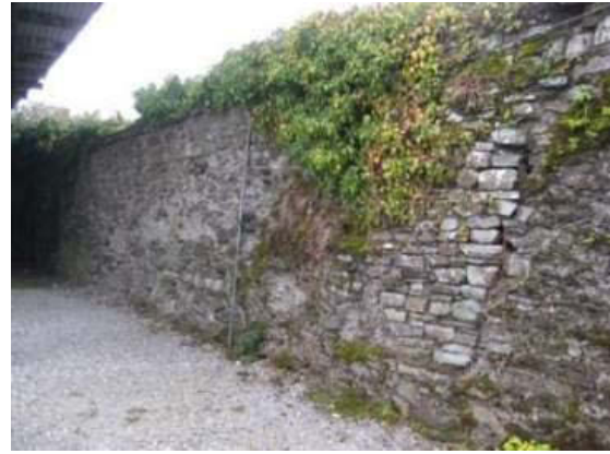
Plate 86: View of wall southwest showing vegetation growth and evidence of rebuilding of wall
