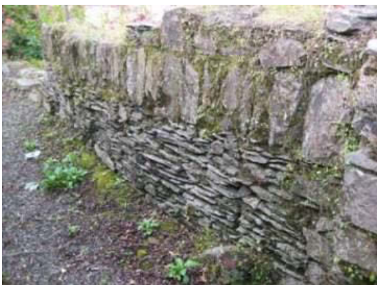
Plate 62: Open joints to east face of west wall
