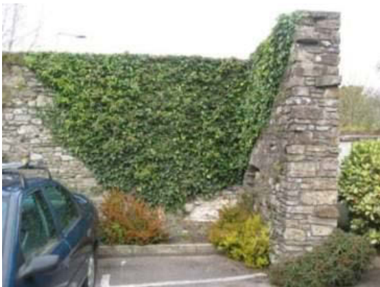
Plate 61: View of east elevation of east wall showing ivy growth
