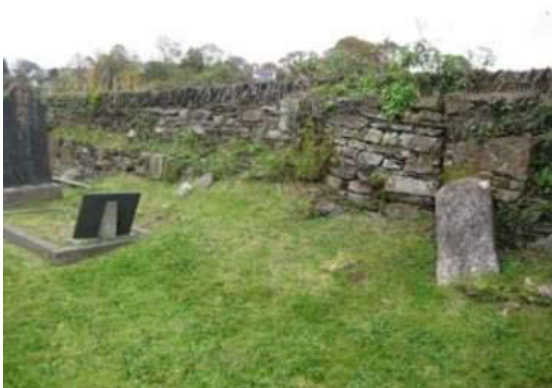
Plate 67: North elevation of wall showing open joints, loss of fabric and biological growth
