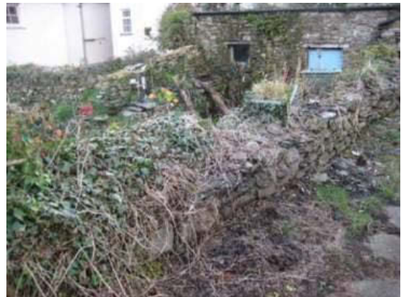
Plate 92: View of section of wall from northeast showing vegetation growth, loose stone and open joints.
