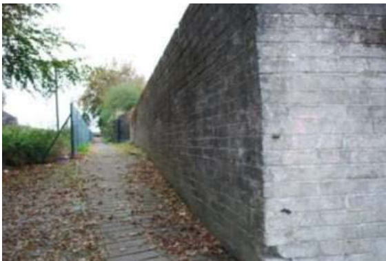
Plate 31: South elevation of east end Section 9. Concrete wall built on line of town wall, looking south-west.
