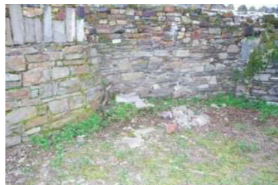
Plate 36: East elevation of southern portion of Section 10, taken from Casement Road. Note later re-build using red brick.
