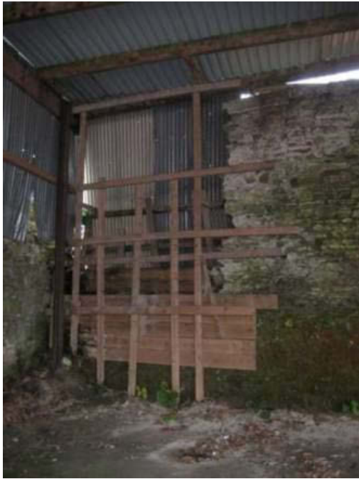
Plate 87: Breach in east-west running section of wall. Note growth of moss to lower reaches of wall
