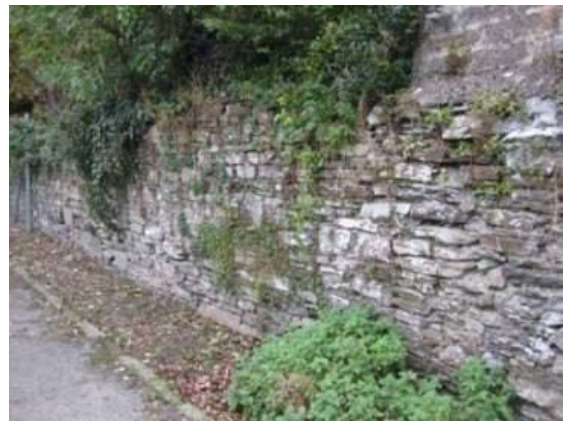
Plate 76: Section towards eastern end showing open joints and biological growth.
