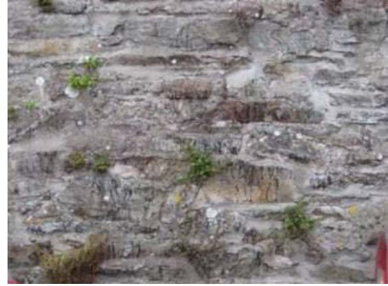
Plate 71: Biological growth and bitumen residue to wall
