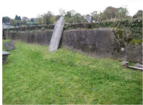
Plate 68: Cementitious render to north elevation
