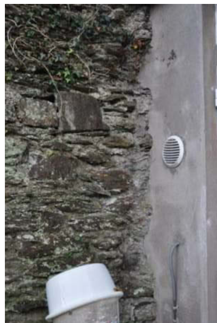
Plate 48: Detail of original masonry where it is adjoined by the dwelling house.
