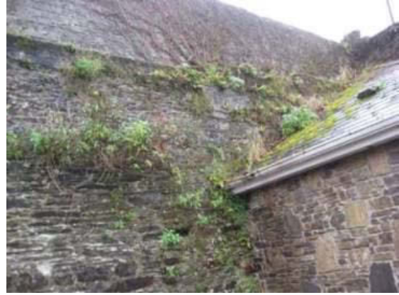
Plate 79: Biological growth to wall. Note concrete block extension to top of wall.
