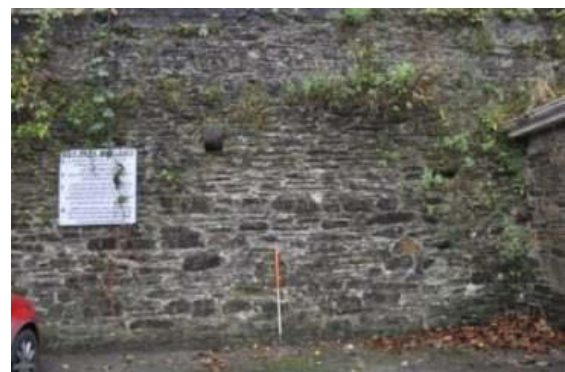
Plate 33: Detail of north-facing elevation at east end of Section 9 within public car park.
