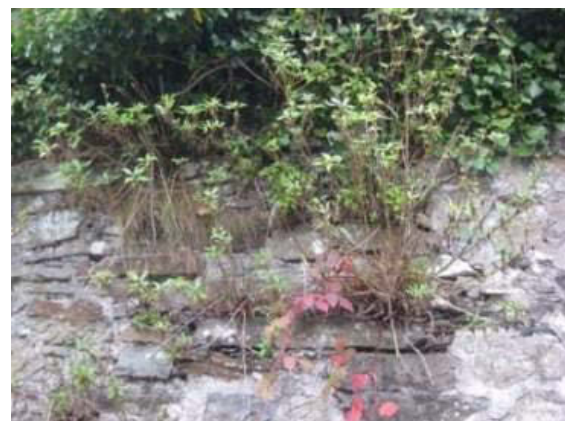
Plate 72: Open joints to wall which have encouraged the growth of plant life
