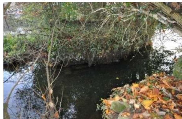
Plate 55: Masonry at and below water level on island in River Bandon, looking south.
