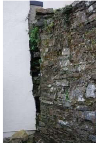
Plate 8: Original town wall (east elevation) where it is abutted by shopping centre building – note collapsed masonry.
