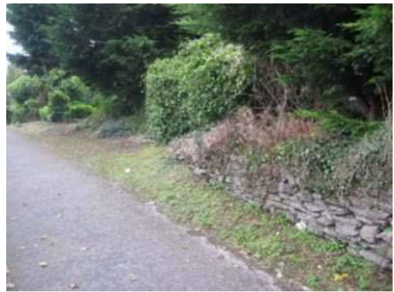
Plate 75: View of wall from southeast showing biological growth, open joints and general poor state of preservation of wall
