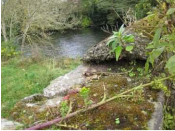
Plate 57: Damaged flaunching to west wall
