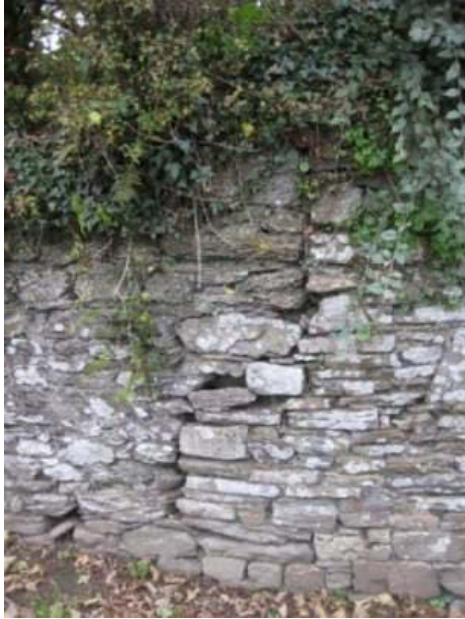
Plate 77: Crack to south elevation of wall
