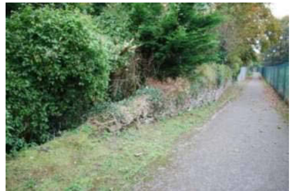
Plate 29: Section 9, possible portion of original upstanding town wall (east of collapsed sections), looking north-east.
