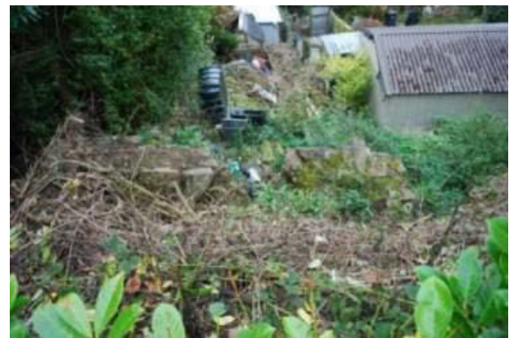
Plate 28: Collapsed wall east of church steps (Section 9), looking north north-west.
