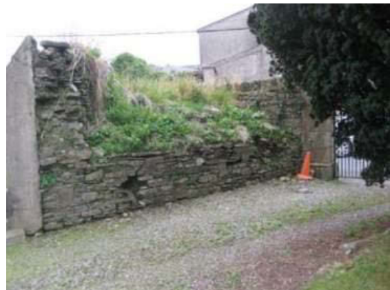
Plate 69: Triangular feature to southeast corner. Note vegetation and build up of detritus to structure
