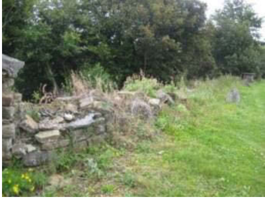
Plate 90: View from southwest showing poor condition of top of wall
