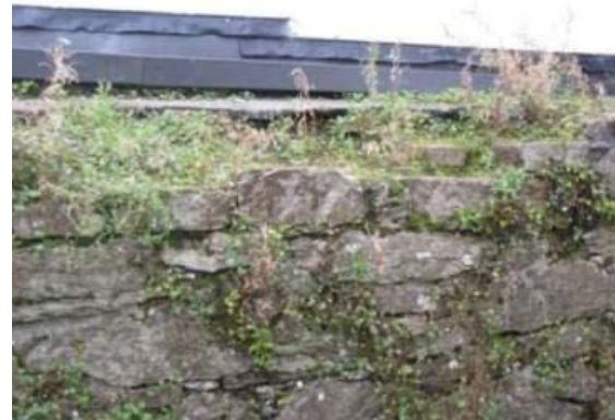
Plate 63: View of section beside Riverside Shopping Centre showing damaged coping and biological growth
