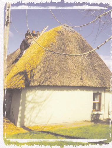
Figure 11. Detail of a hipped roof, Shandrom, near Charleville, North Cork. CCC No 5.
