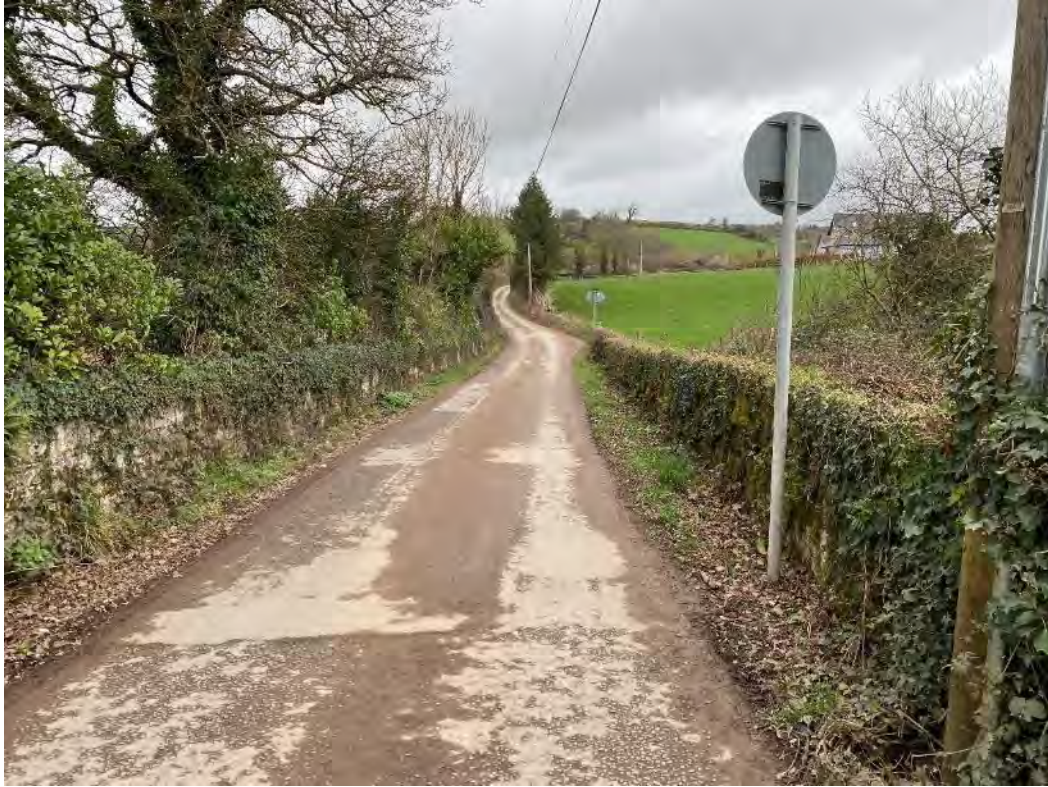
Plate 43: Portion of local road for upgrading at the eastern end of the UEA scheme
