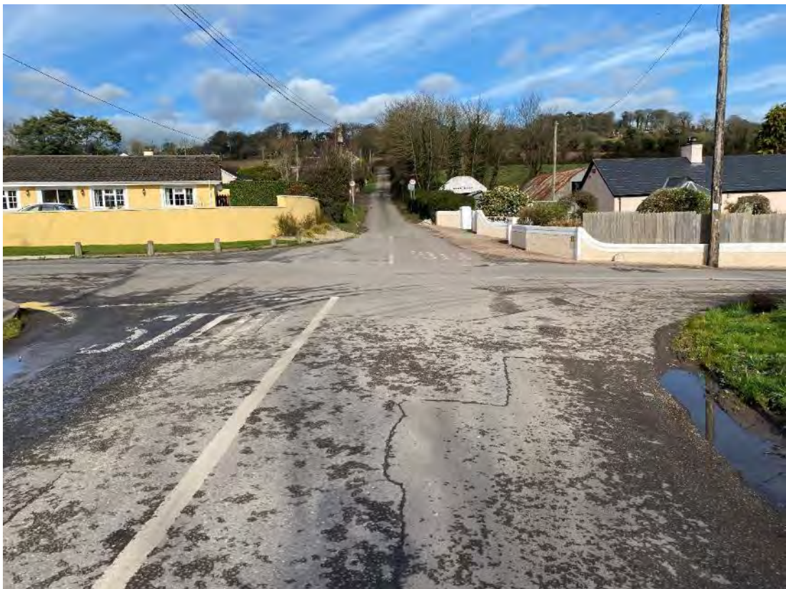
Plate 46: Cross roads for upgrading at the far north-western portion of the UEA scheme
