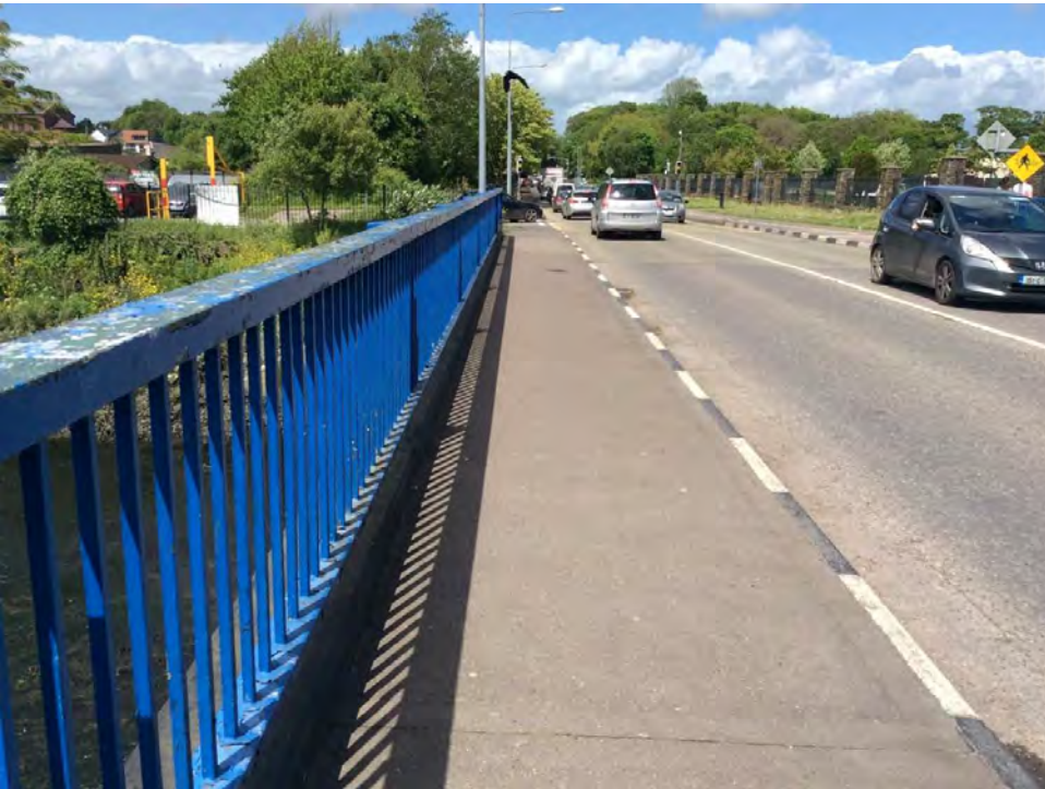
Plate 10: Existing modern road bridge over Owenabue River just outside eastern site boundary, looking N.
