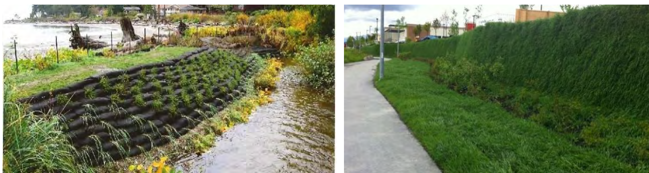
Image 5.8: Example of steepened slope reinforced soil embankment (left before growth, right after growth)
