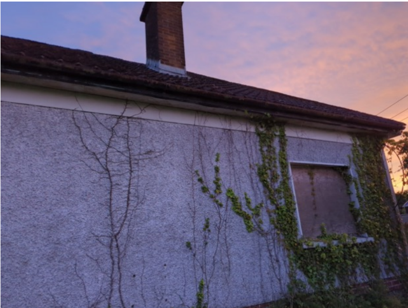
Plate 4. Gable (1) with boarded up window minor with ivy growth and intact wooden fascia
