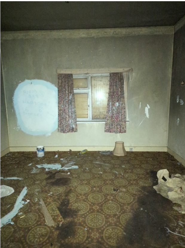
Plate 8. Building interior showing signs of dampness
