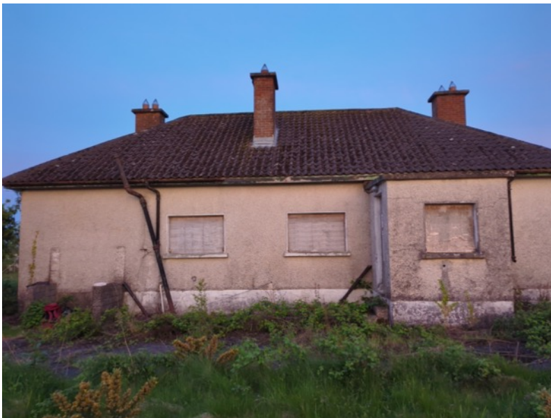
Plate 2. Rear of dwelling with boarded up windows and wooden faces in relatively good condition
