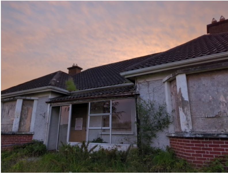
Plate 1. Front of disused dwelling with broken windows on porch
