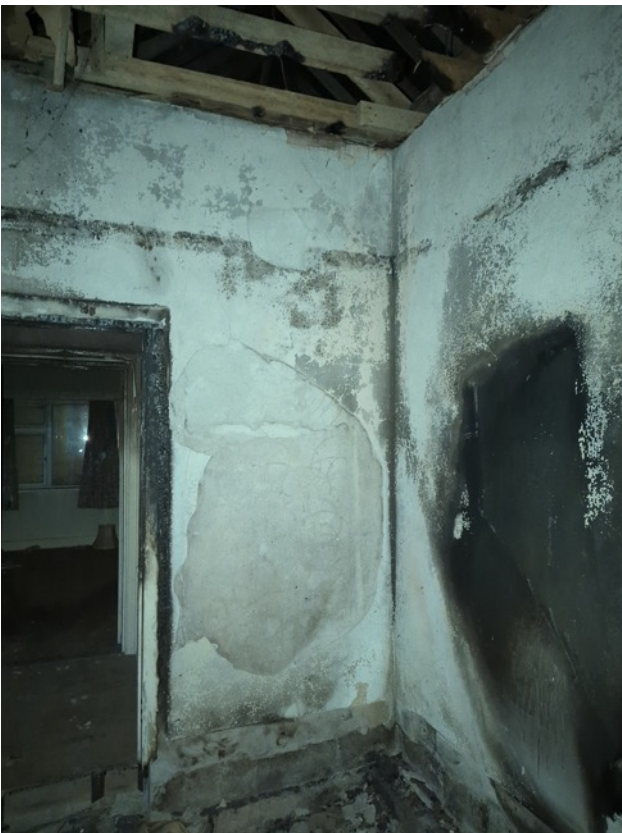
Plate 6. Fire damage within building interior
