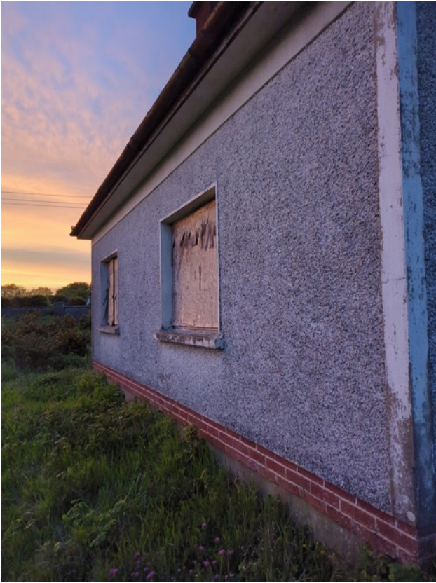
Plate 5. Gable (2) with boarded up windows and intact fascia
