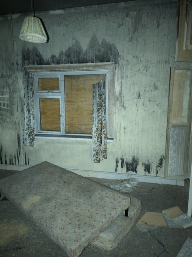
Plate 9. Building interior showing signs of dampness
