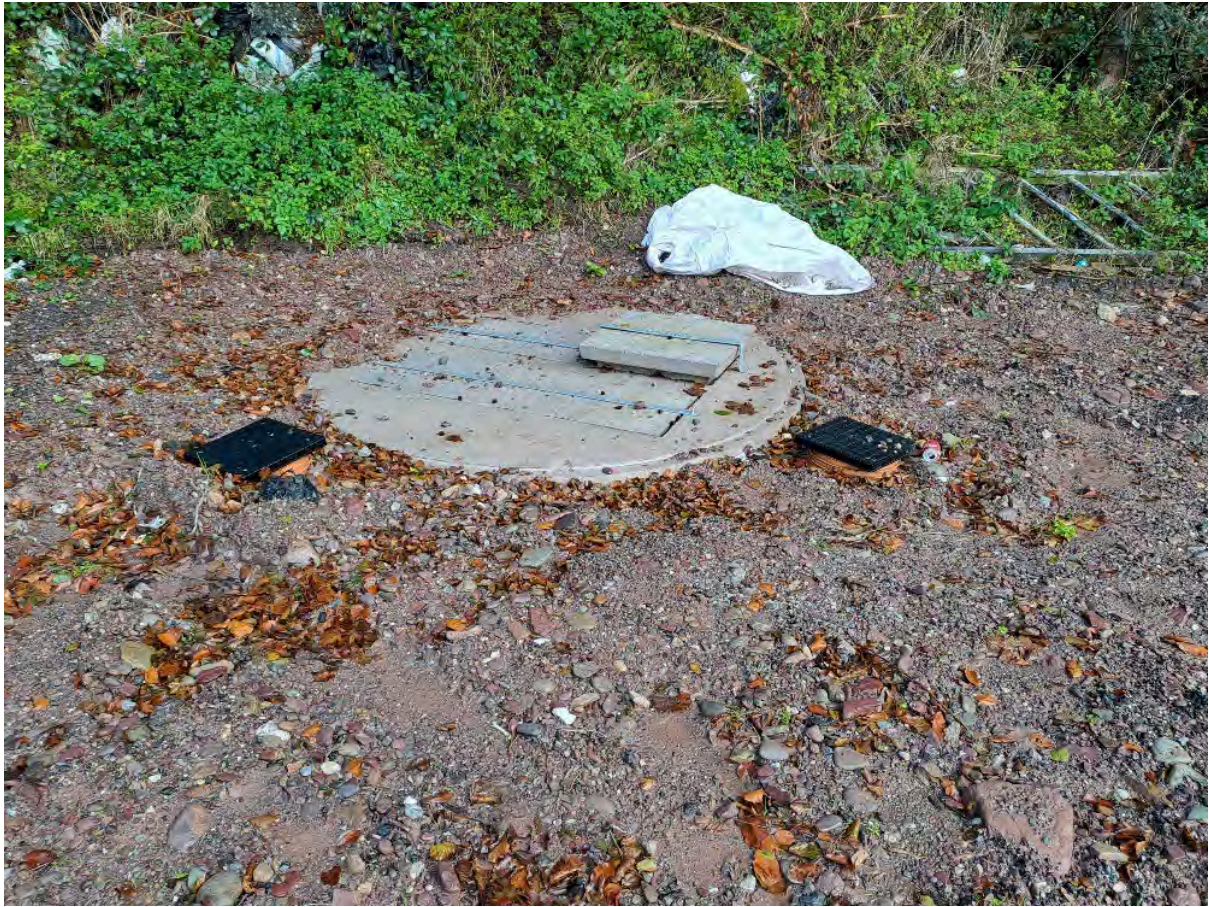
Photo 10. No evidence of discharge from “septic tank”.
