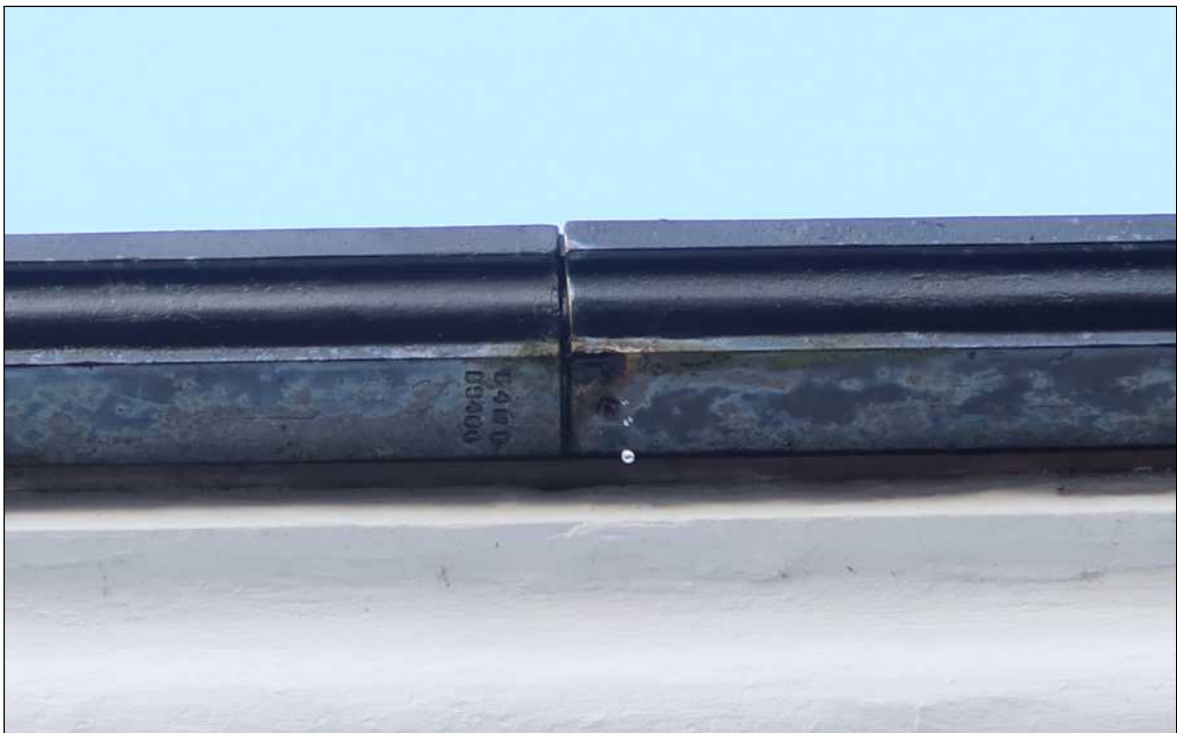
• Fig 78. Leaking gutter junctions in places (over Eastern wing South elevation.) Corrosion evident also.
