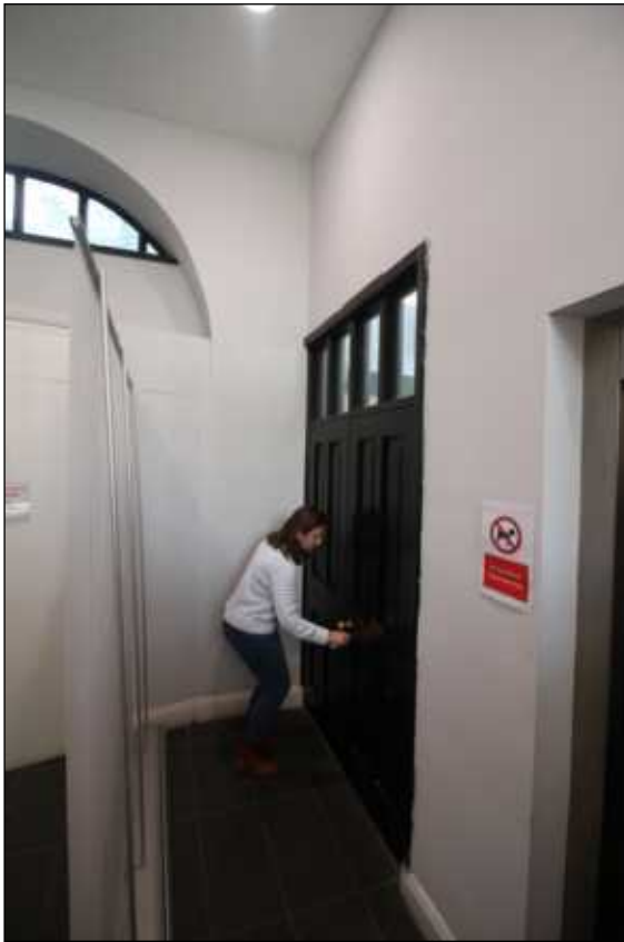
• Fig 66 Entrance to plant room.
