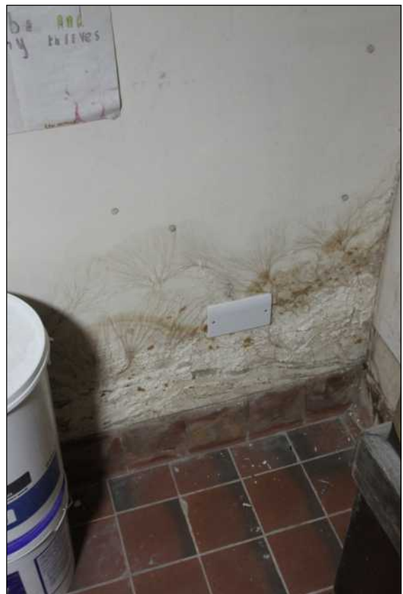
Fig 69. Damp issues in rear rooms.
