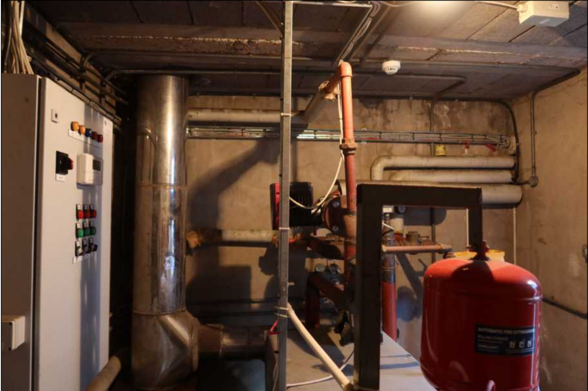
• Fig 73. Boiler room No. 13.
