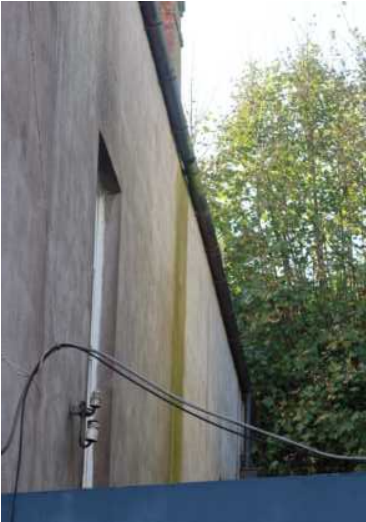
• Fig. 83. Leaking rear gutters.
