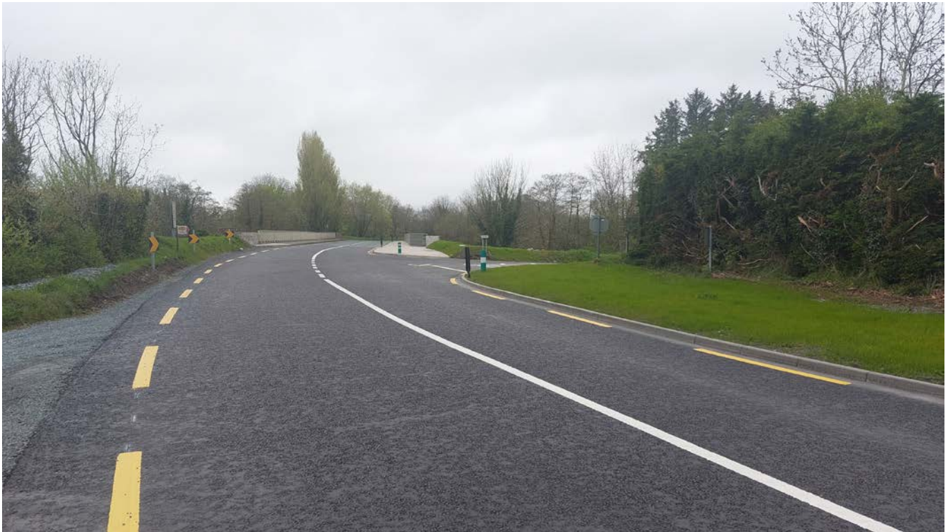
Photo of Works undertaken on the Mallow–Millstreet Road to improve sightlines at the junction near Keale Bridge.
