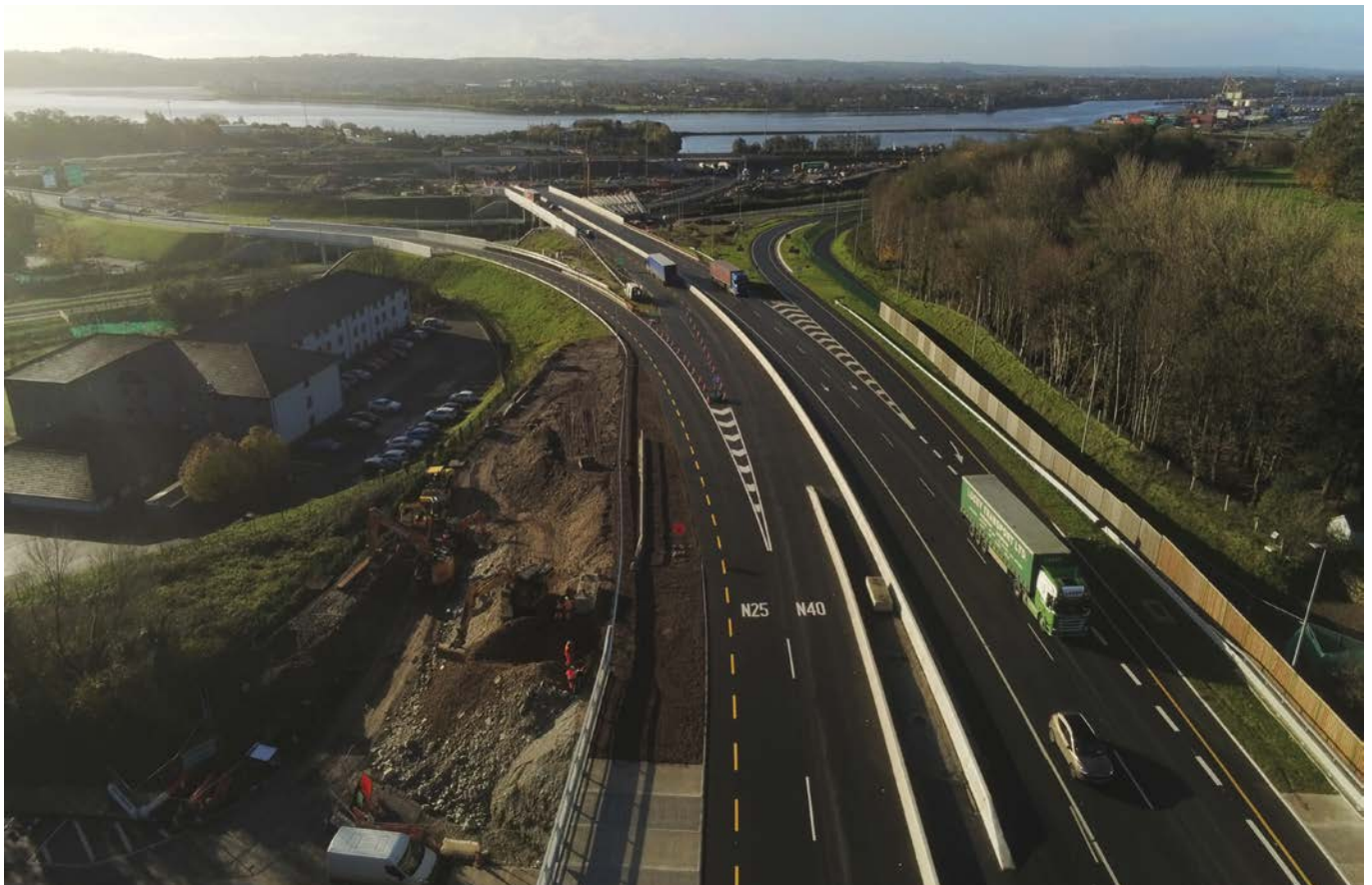
The M8 Southbound approach to the Dunkettle Interchange showing new structures over the Cork – Middleton Railway line which will provide free flow access to the N40 via the Jack Lynch tunnel and free flow access to the N25 Eastbound.
