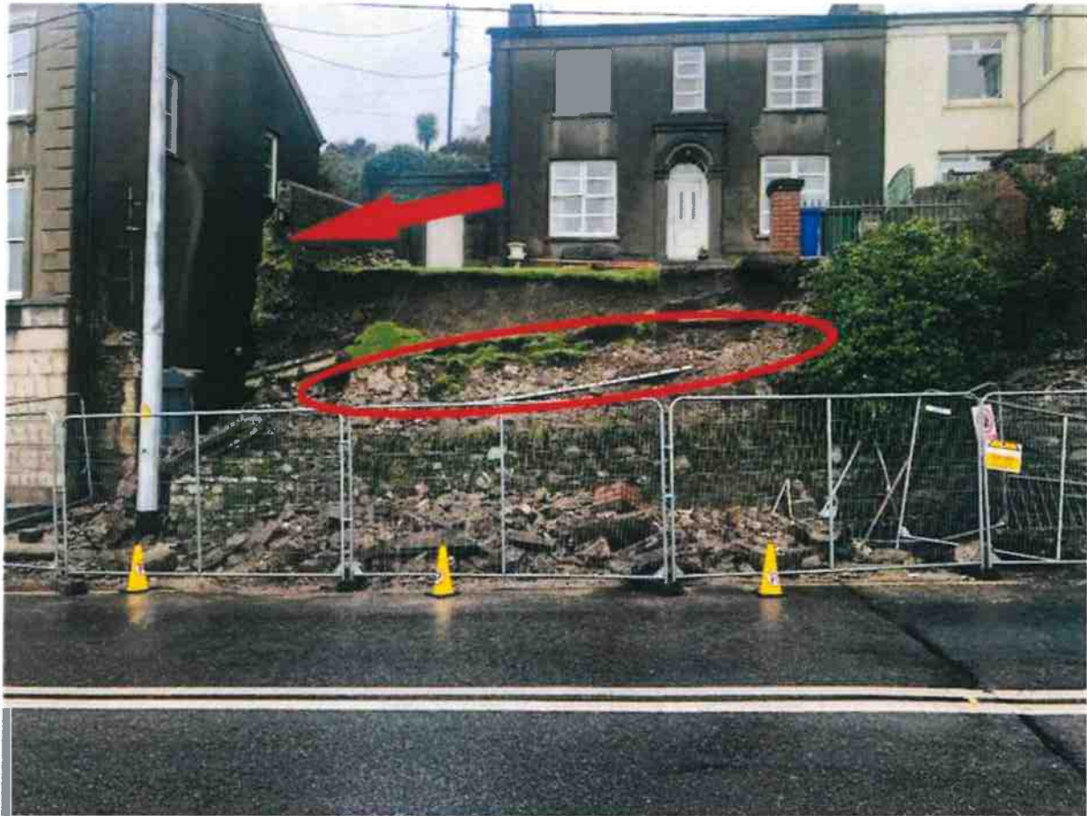
Figure 9 Retaining Wall Collapse
