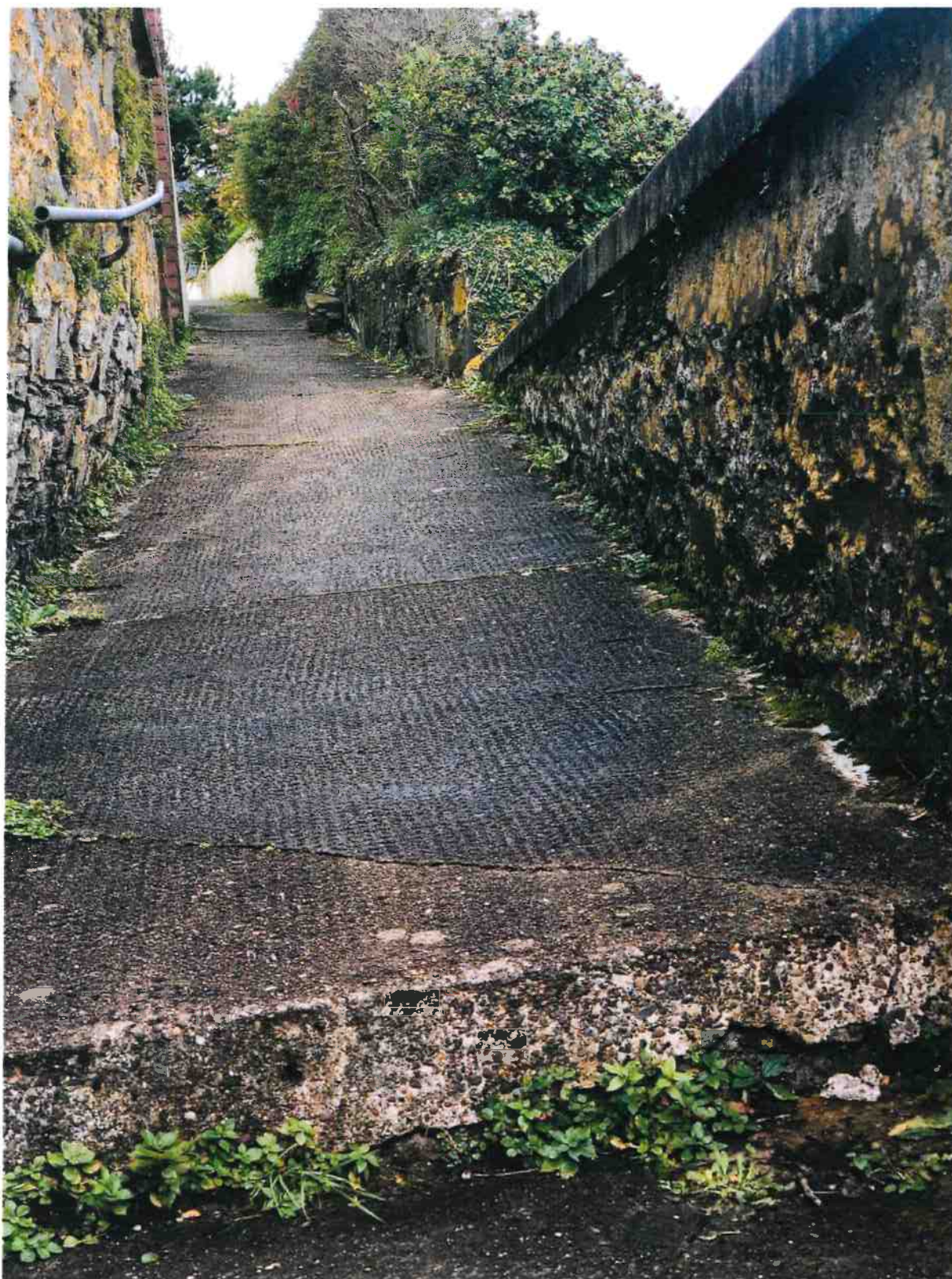
Figure 3 Walls A (Bulging, Left) and C (Right)
