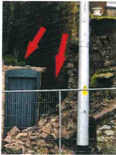
Figure 10 Damage to Neighbour's Side Access
