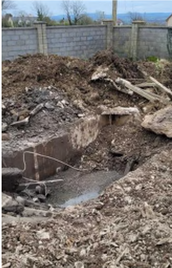
Redundant Septic tank to rear of no. 19 & 20
