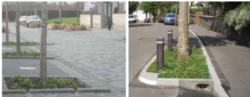
Figure 11: Examples of tree pits in isolated green planters from the CIRIA SuDS Manual
