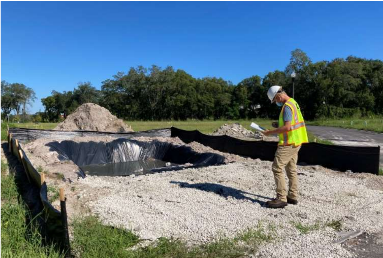
Figure 7 - Concrete Truck Washout Area with Impermeable Liner
