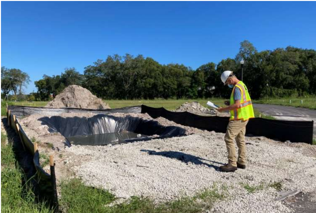
Figure 7 - Concrete Truck Washout Area with Impermeable Liner
