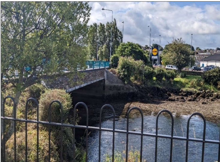
Plate 4.5 Bridge at eastern boundary of the proposed works site on which the R612 lies (TII Bridge ID: CC-R612-001.00).
