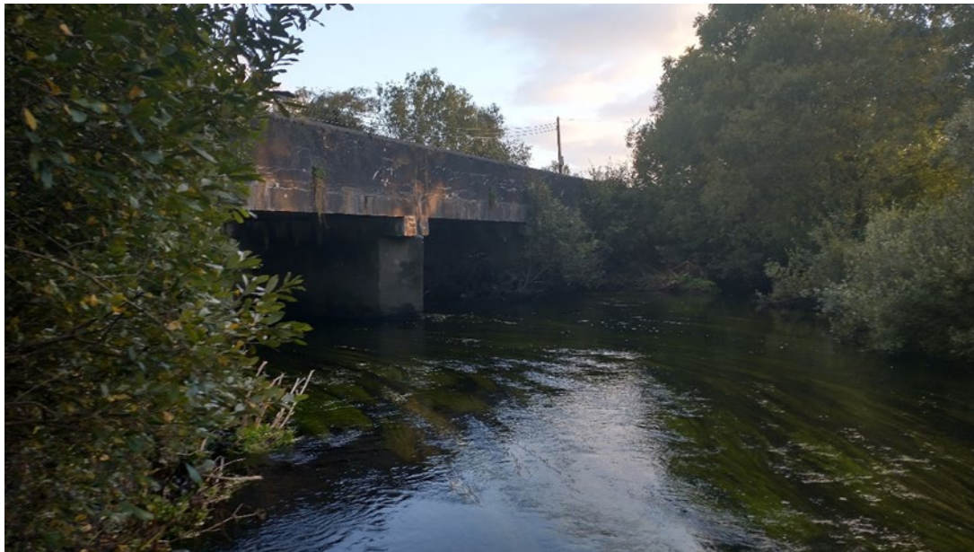
Plate 2-4: View of arches visible from upstream location (arches 3-5). Arches 1, 2 and 6 are blocked by dense vegetation from the upstream location.
