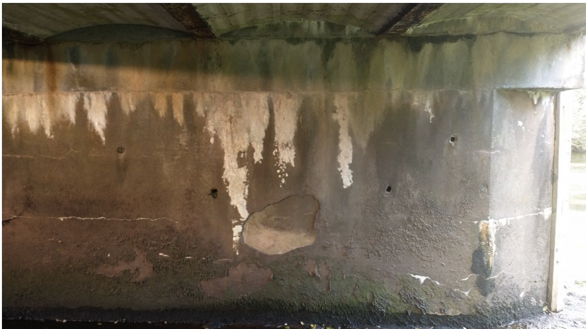
Plate 2-1: Holes in west-facing pier in arch 6 (western arch).
