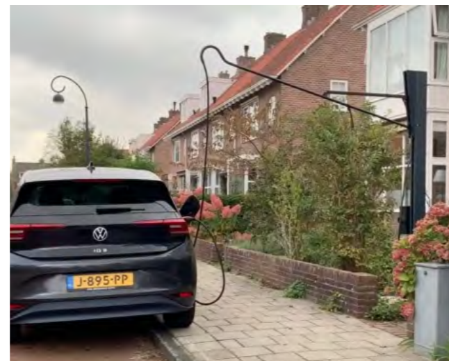
Private charging to cross pavement for on-street parking
