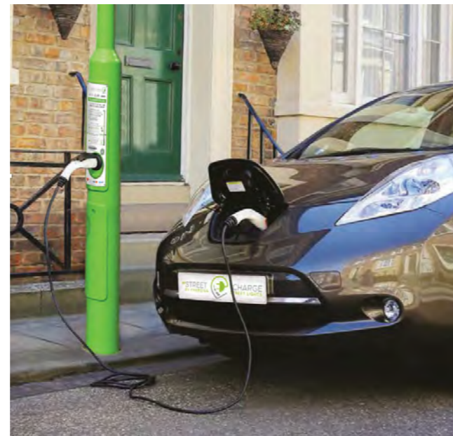
Charging incorporated in to light columns
