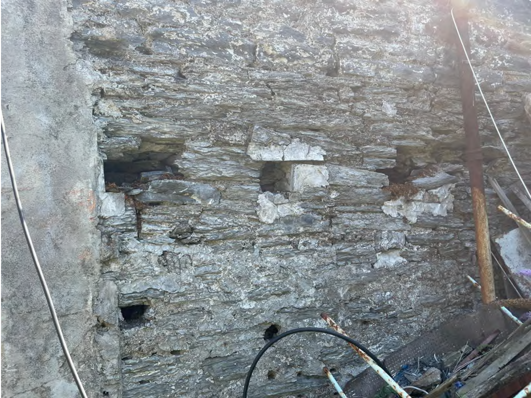
Photograph No. 7 – Lintel Openings
