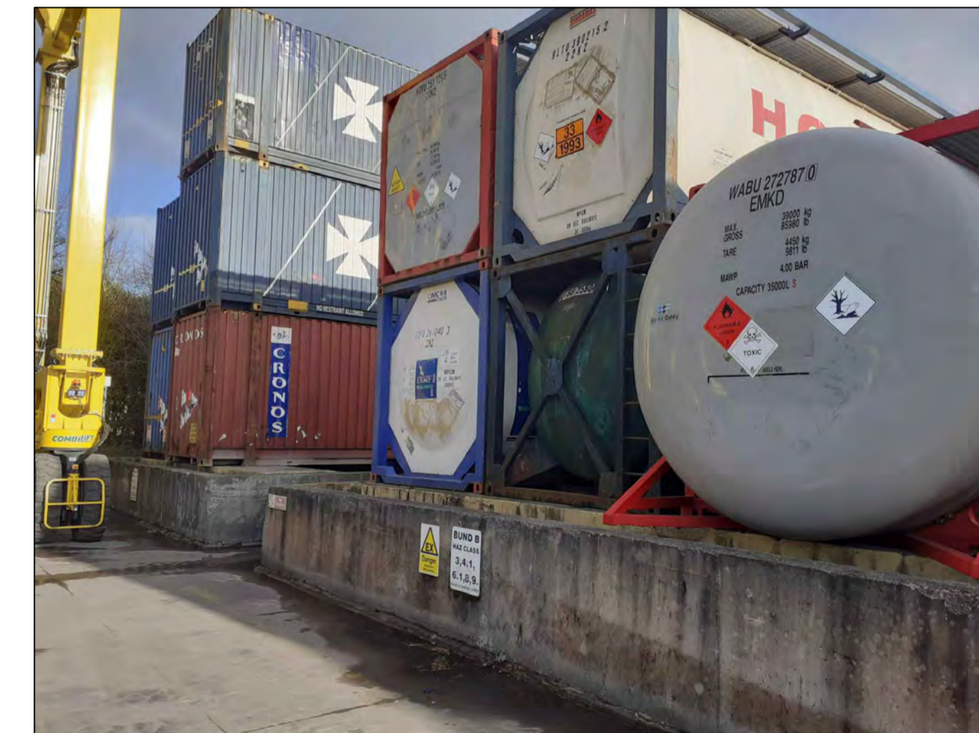
PHOTOGRAPH No 1, EXISTING BULK STORAGE TANKS BUND B (See Site Plan over for photograph location)
