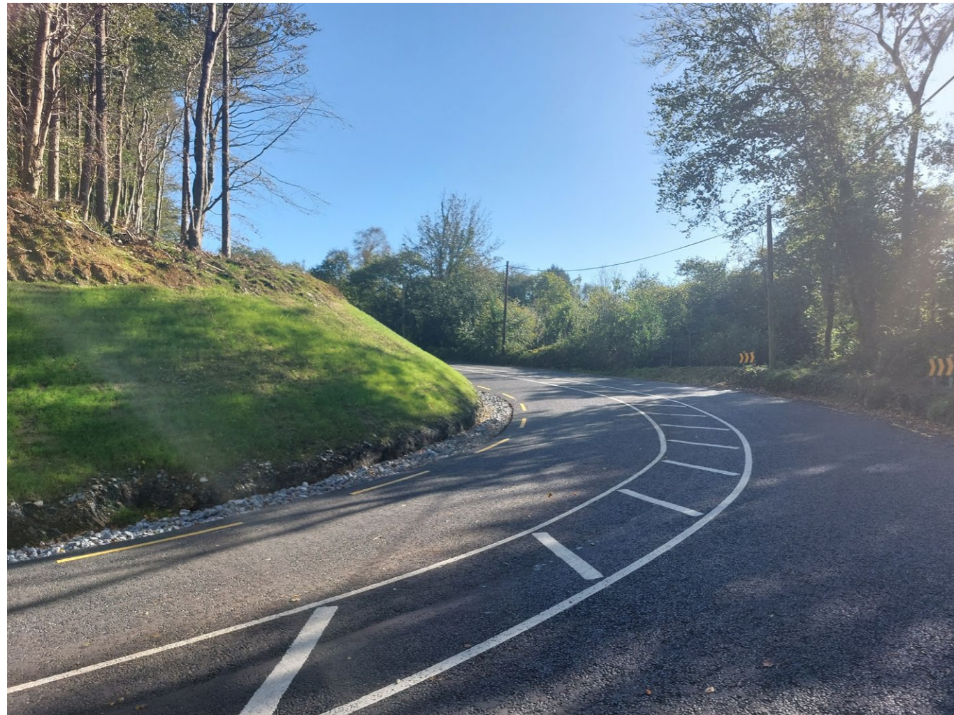
Works undertaken on R605 Innishannon to Kinsale Road at Shipool to widen the road and improve forward visibility.
